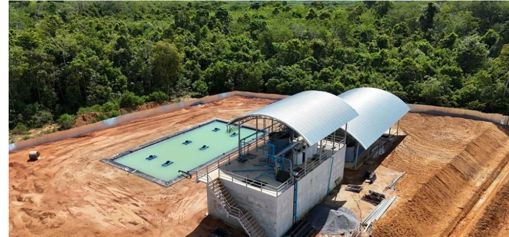
Wastewater treatment 65 CBM/day
