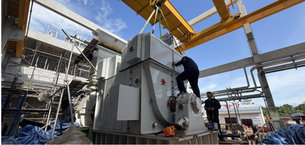
Turbine and generator
