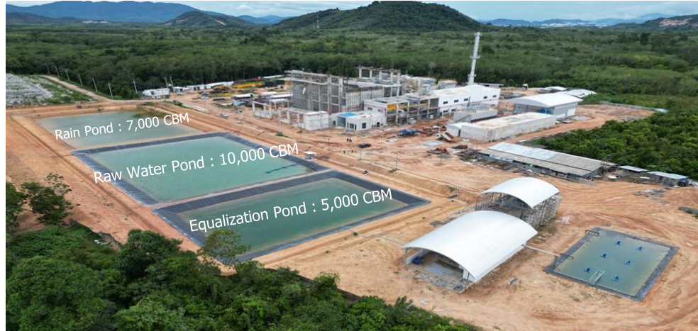
Pond : Rain water retention, raw water, equalization
