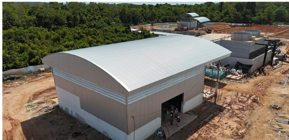
Water treatment capacity Service 45 cum, RO 15 CBM, DI 4 CBM/hr
