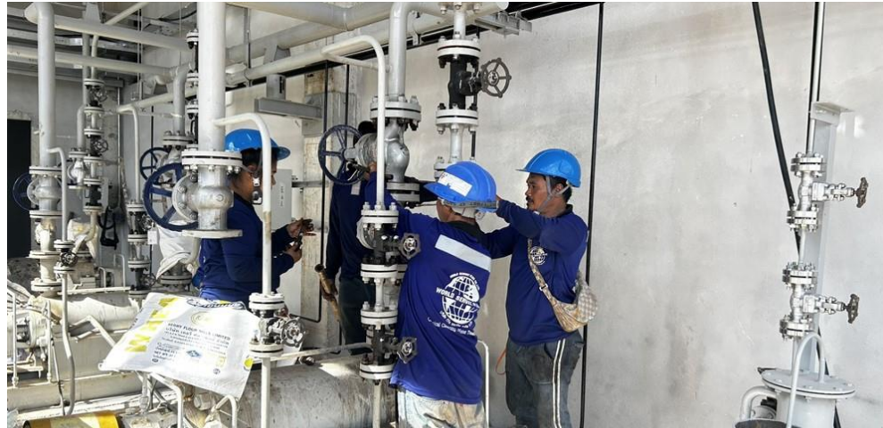
Chemical injection system installation for feed water
