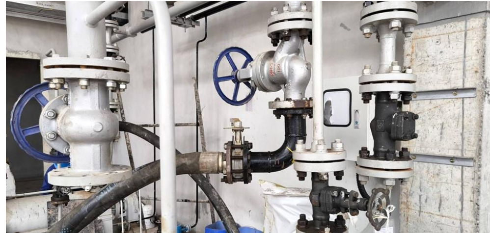
Chemical injection system installation for feed water
