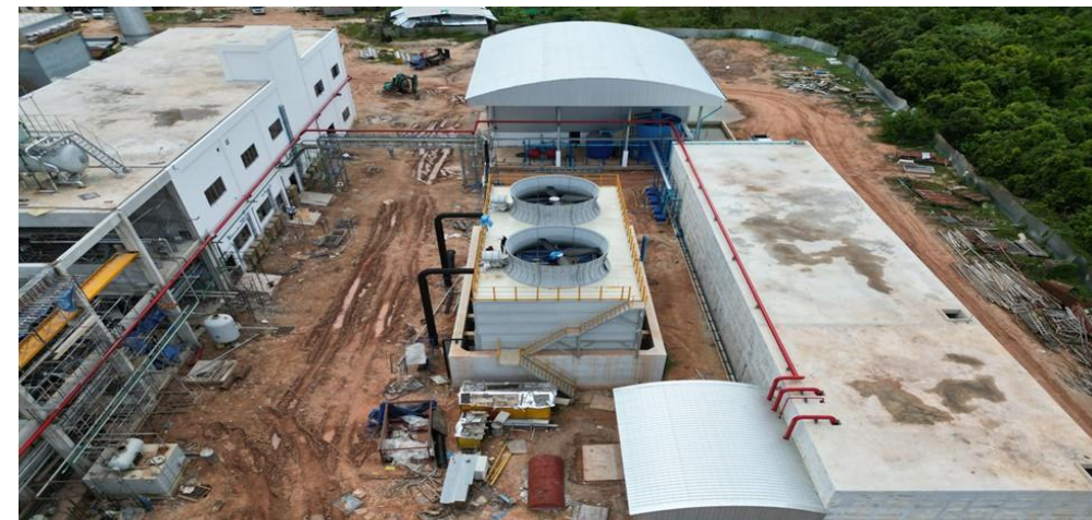
Cooling tower 40 CBM/day and Service tank 2,000 CBM
