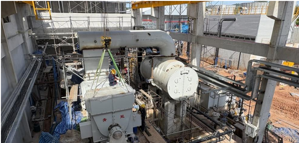
Turbine and generator
